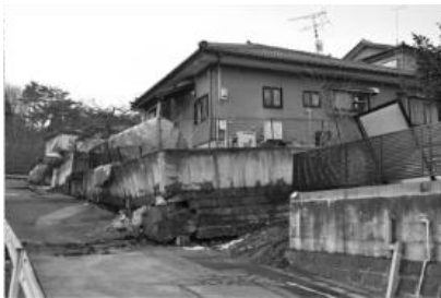
Residential Land damage damage (Oritate, Aoba Ward)
