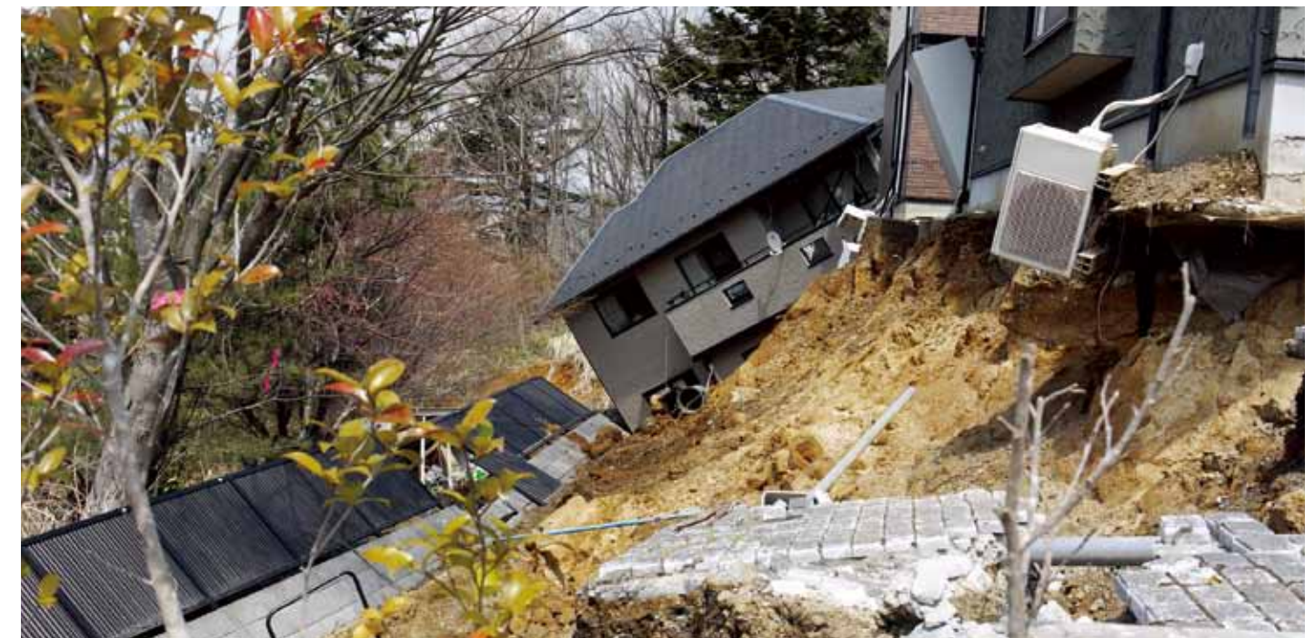
Damage to a hillside suburban residential area (Seikaen, Aoba Ward)
