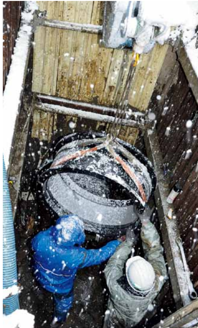
Recovery work on damaged water pipes continued in heavy snow. Water supply was restored on March 29, 18 days after the disaster.
