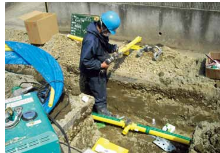
Construction work took place to replace damaged gas pipelines with quake-resistant polyethylene pipelines.
