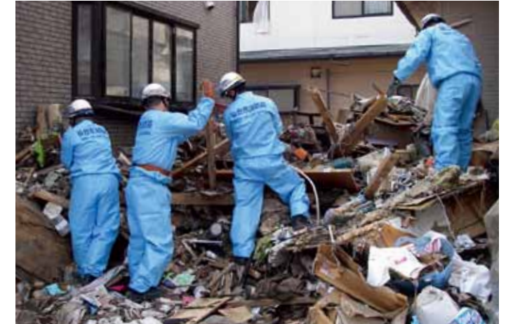
Search and rescue efforts focusing on collapsed houses (April 16, 2011)
