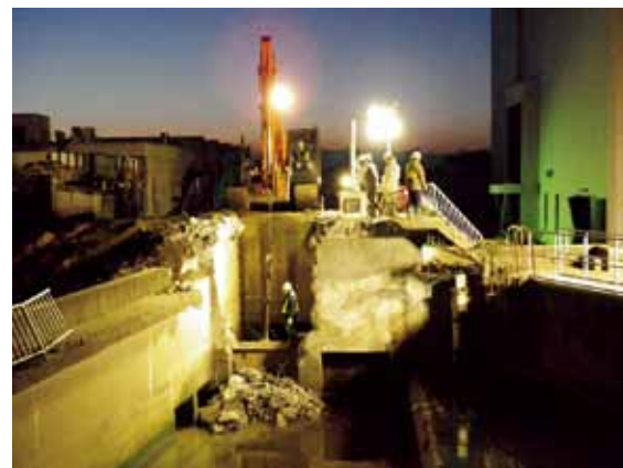
On March 12, 2011, Minami-gamo Purification Center dedicated all of their efforts to resume sewage treatment of their 716,000 customers. Workers can be seen removing debris from the water discharge gate (March 16, 2011).
