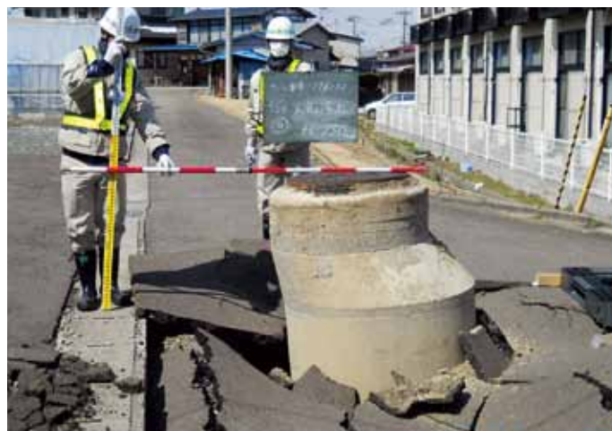
The earthquake caused manholes to protrude from the ground.
