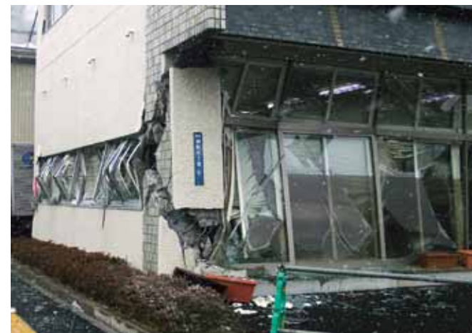
A building damaged by the earthquake
