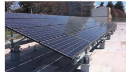
Solar panels installed on the roofs of schools and other facilities that will function as evacuation centers in disaster situations.
