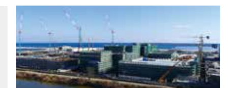
Restoration work on the Minami-Gamo Wastewater Treatment Plant proceeded at full speed. (January, 2015)
