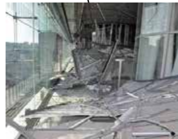
Damaged public facilities
